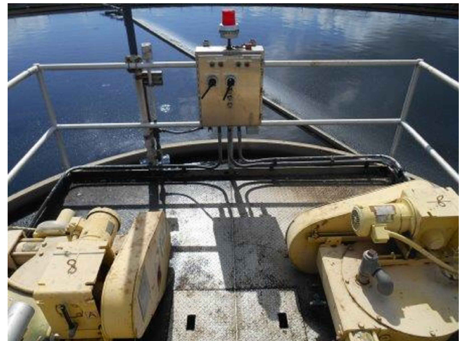
PRIMARY CLARIFIER NO.4 PHOTOGRAPH B
