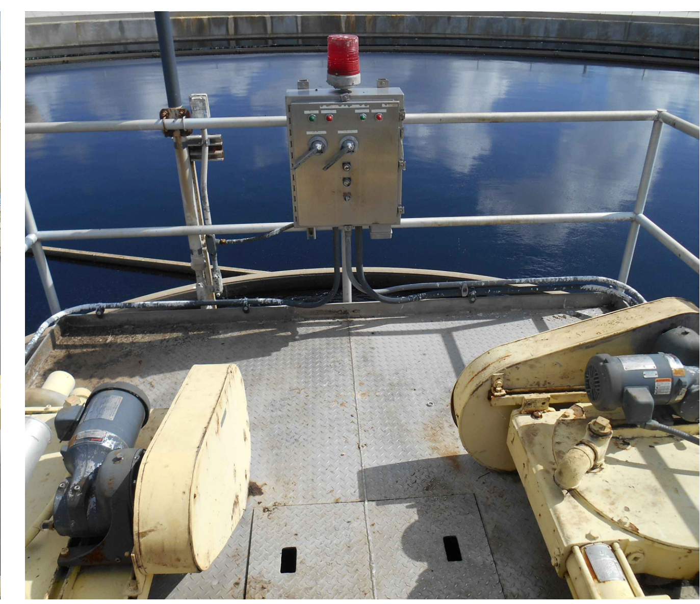
PRIMARY CLARIFIER NO.6 PHOTOGRAPH B
