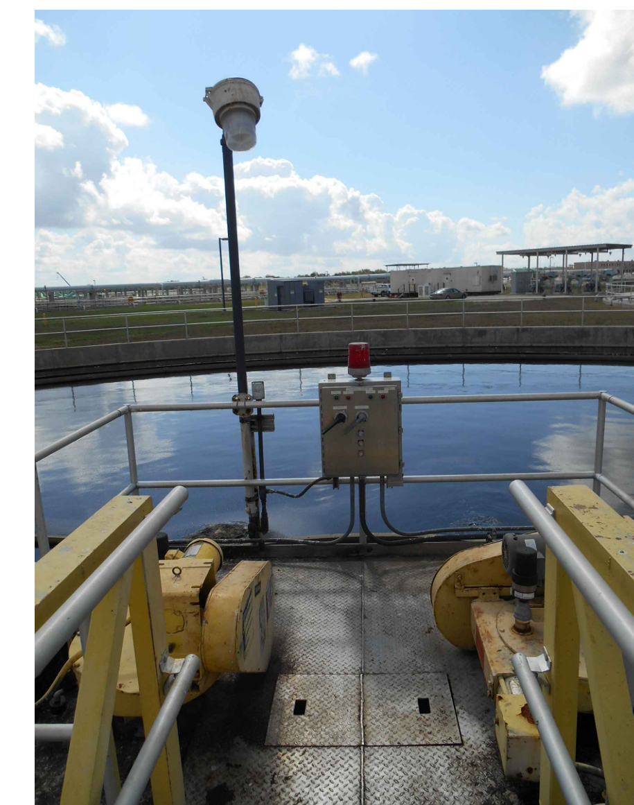
PRIMARY CLARIFIER NO.8 PHOTOGRAPH B
